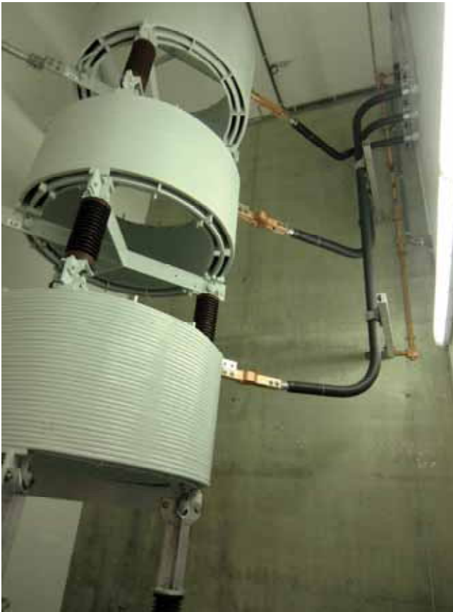
Connection to the current limiting reactors
