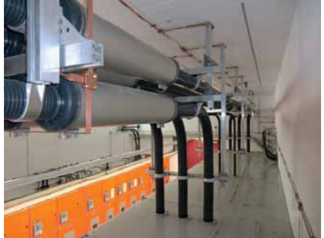
Connection to the switchgears
