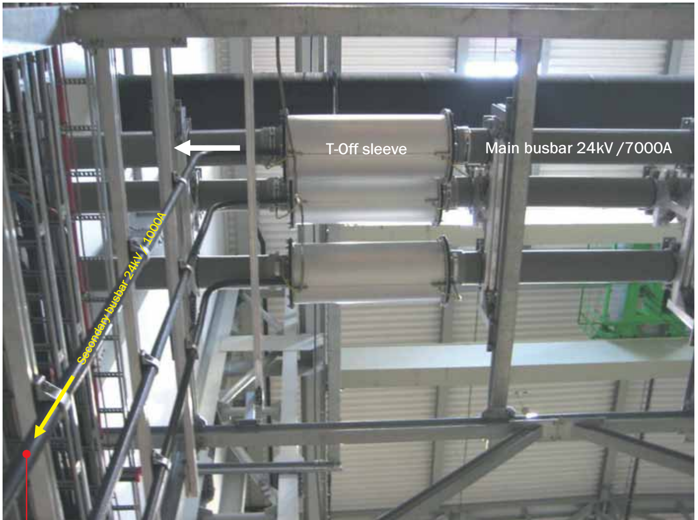
Connection to the auxiliary transformer
