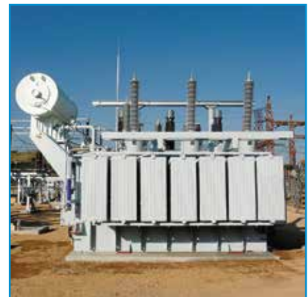
Power Transformer equipped with Moser Glaser Bushings
