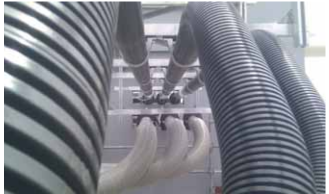
Busbars through the wall
