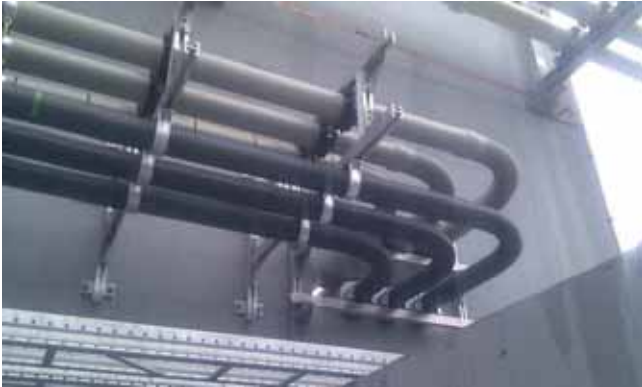
Busbars through the wall
